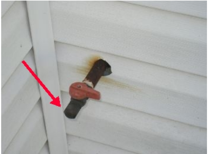
Gas connection for outdoor grill
