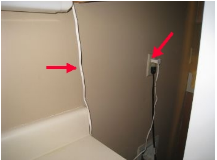
Extension cord used for permanent wiring in kitchen
