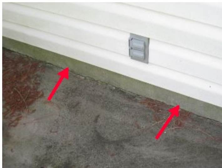
Caulking recommended at patio
