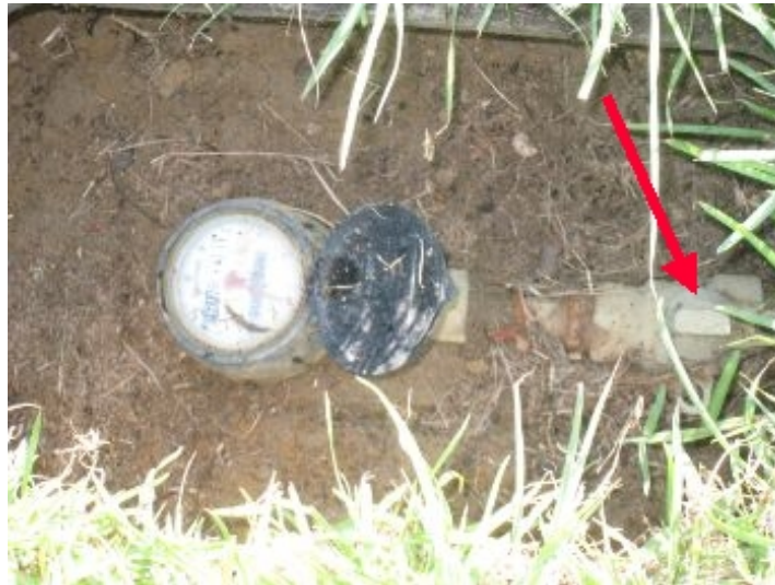
Water meter and main shut-off valve
