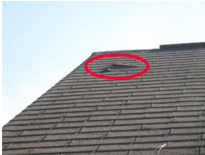
Roof repair required
