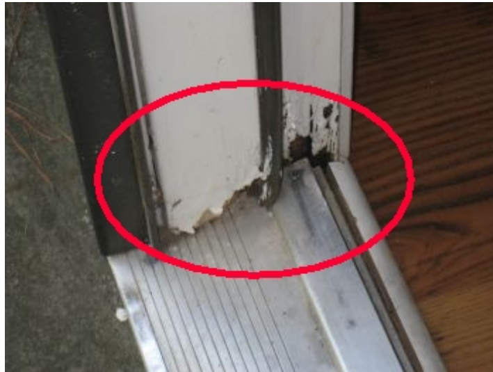
Water damage at bottom of rear door
