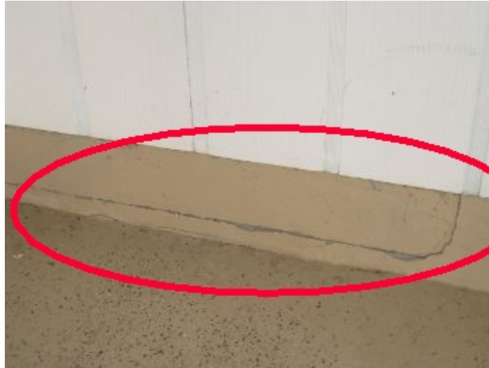
Apparent impact damage in garage
