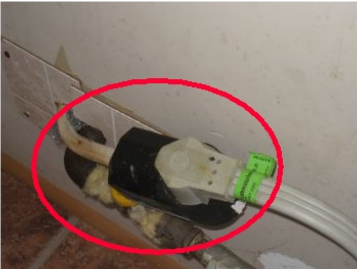
Improper wiring for range
