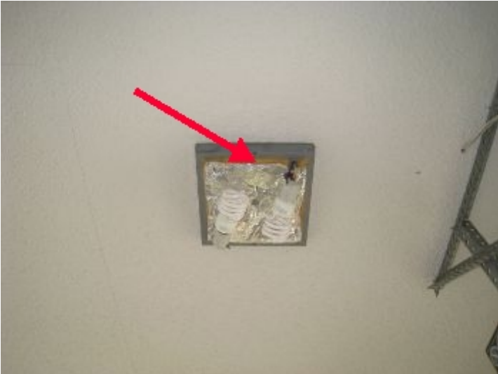
Missing fixture cover in garage
