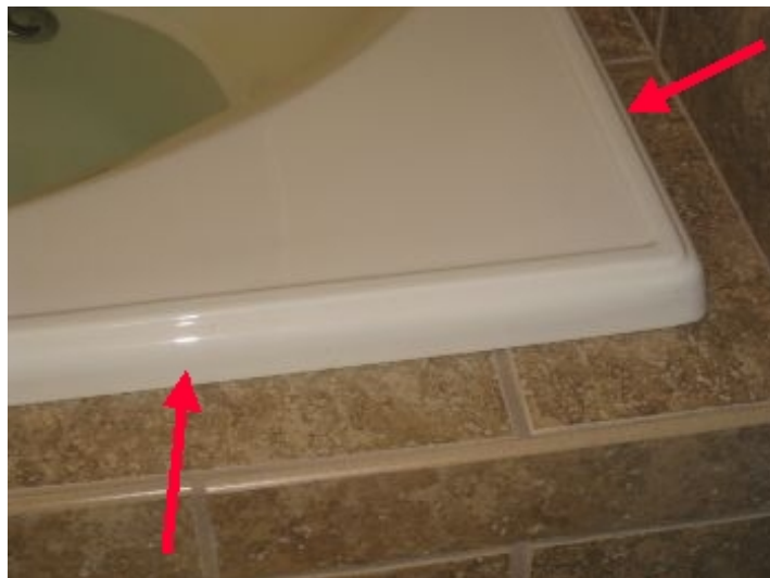
Caulking recommended at whirlpool tub
