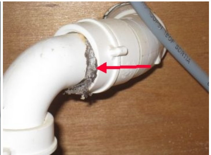
Leak in hall bathroom drain
