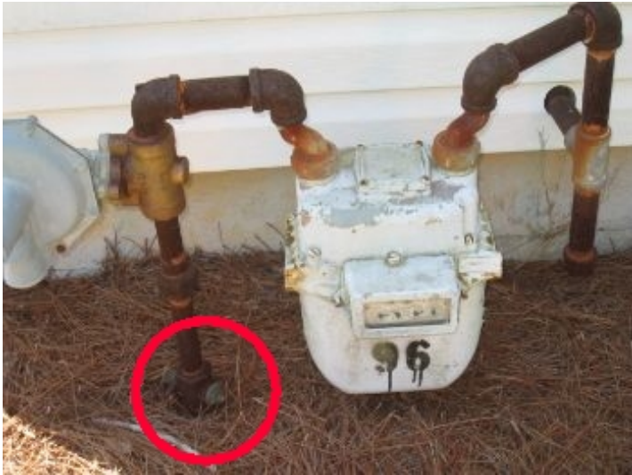
Gas meter and main shut-off
