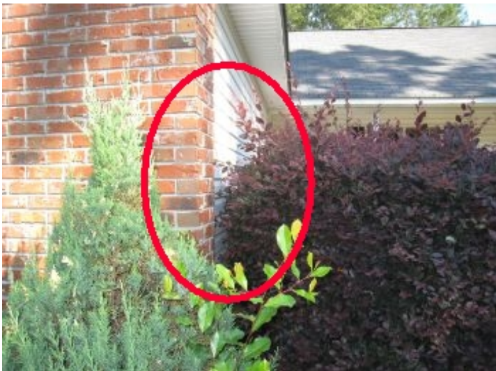
Vegetation against structure
