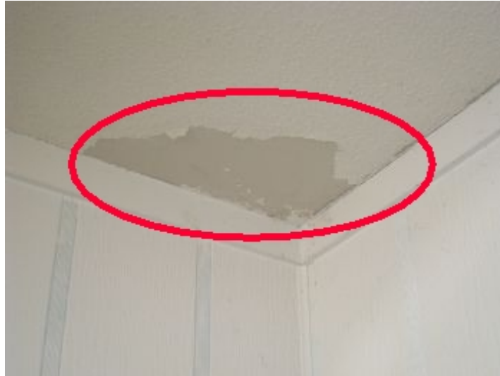
Ceiling damage in garage
