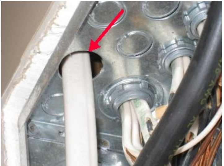
No cable protection in opening
