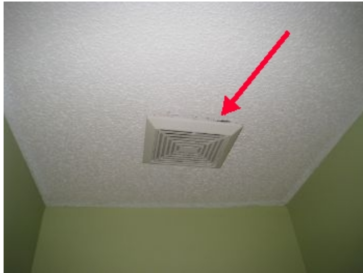
Unsecured exhaust fan (master bathroom)
