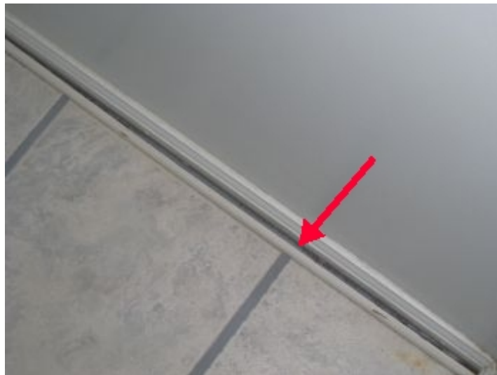
Loose shoe molding in hall bathroom closet
