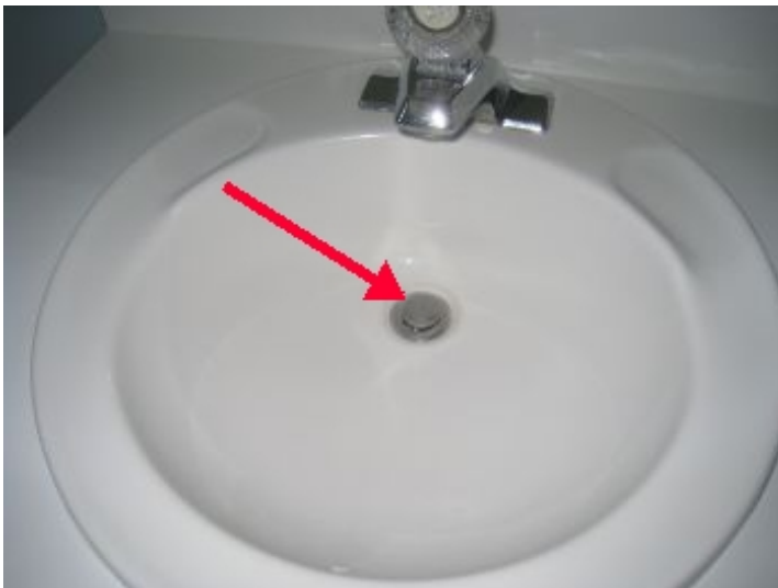
Inoperable pop-up drain in hall bathroom
