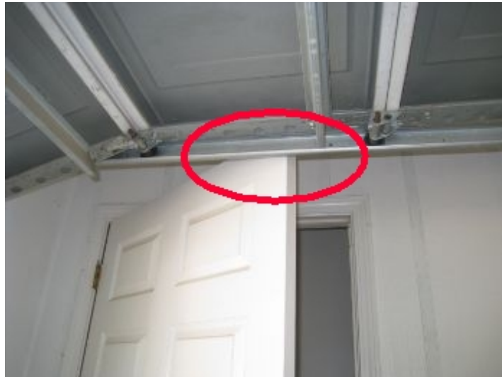
Utility room door / garage door interference
