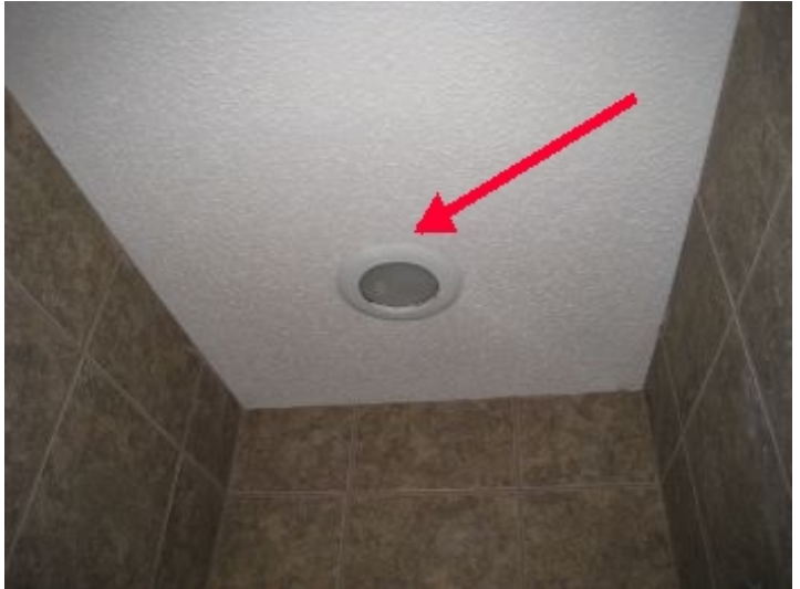
Inoperable light in master bathroom shower
