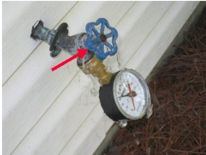
Leaking hose bib
