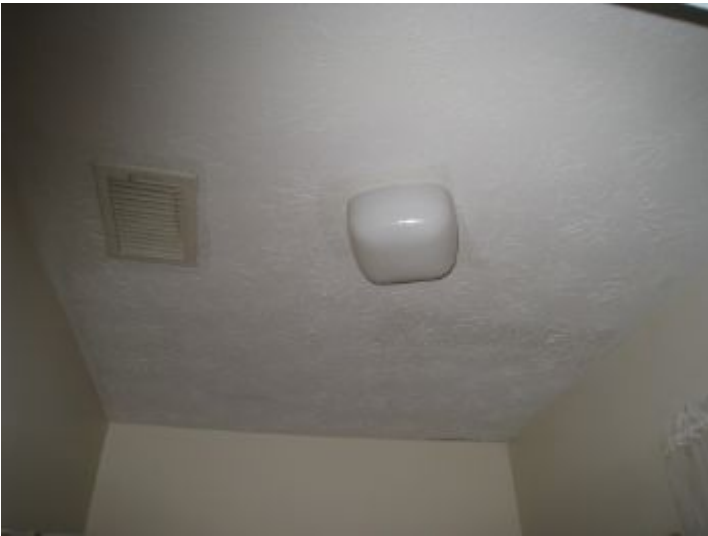
No exhaust fan in master bath
