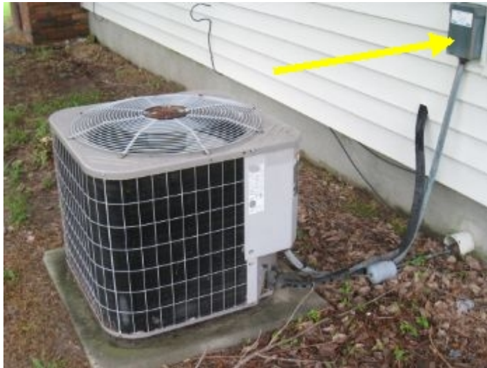
Heat Pump compressor and local disconnect
