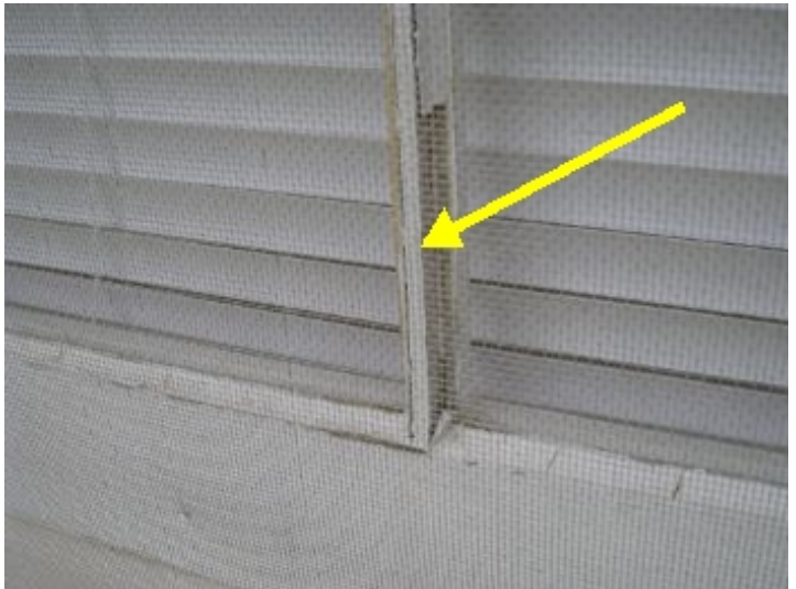
Failing caulk on windows
