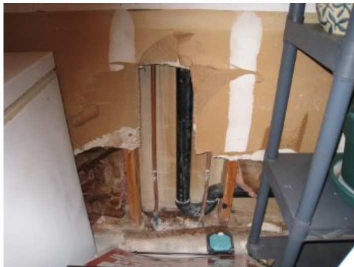
Holes in wall - utility room
