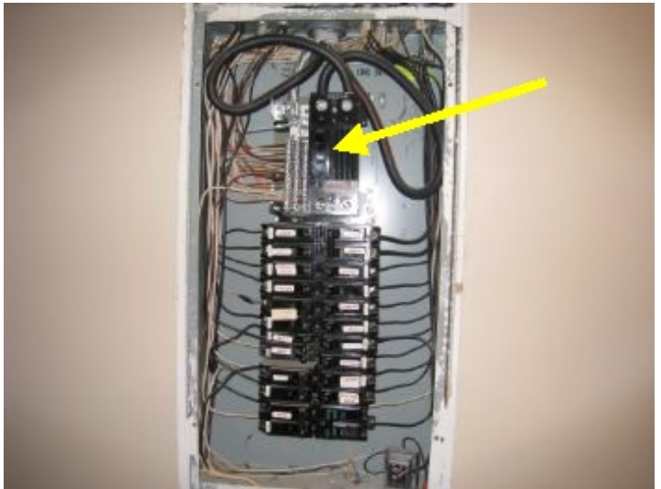
Interior of service panel and main breaker
