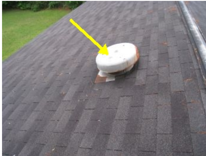
Powered roof ventilator
