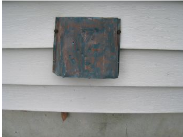
Dryer vent at rear of house
