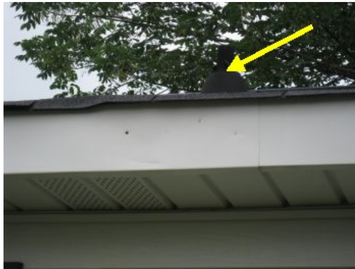
Deteriorated rubber boot around plumbing vent
