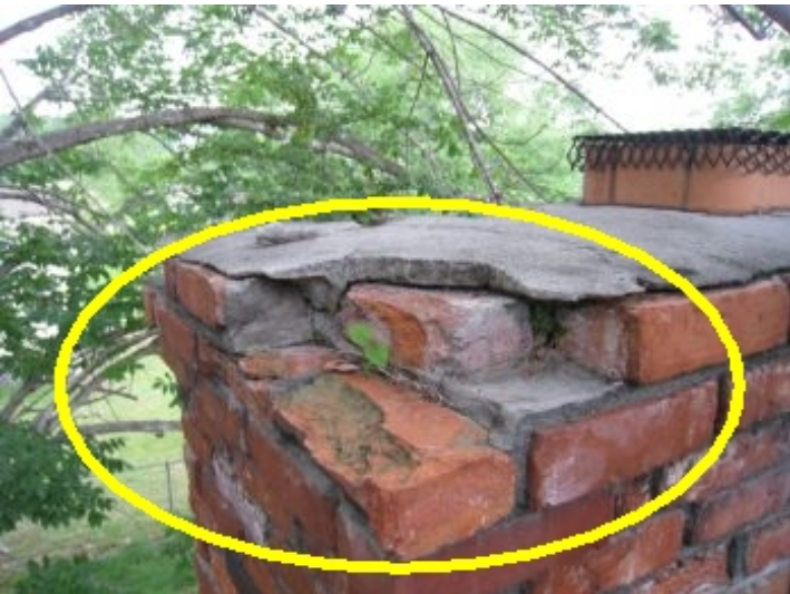
Deterioration at top of chimney
