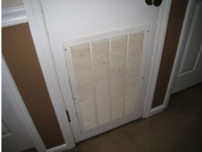
Poorly constructed return air filter arrangement
