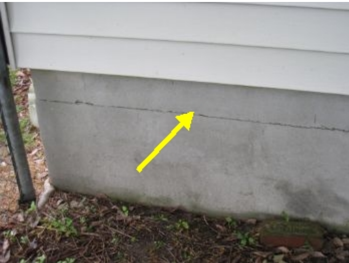
Minor foundation crack
