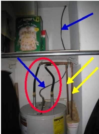
Unsupported piping (yellow), no shut-off valve(red), and loose wiring(blue)
