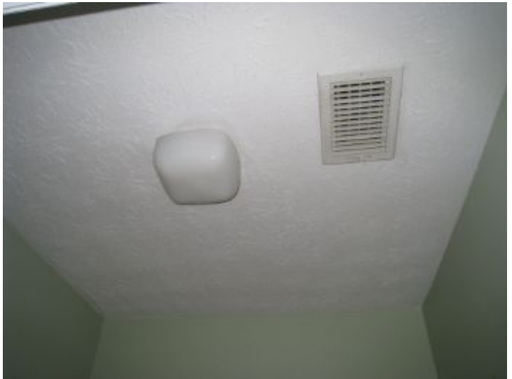
No exhaust fan in hall bath
