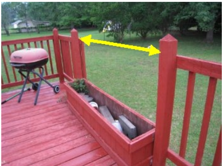
Missing railing at rear of deck
