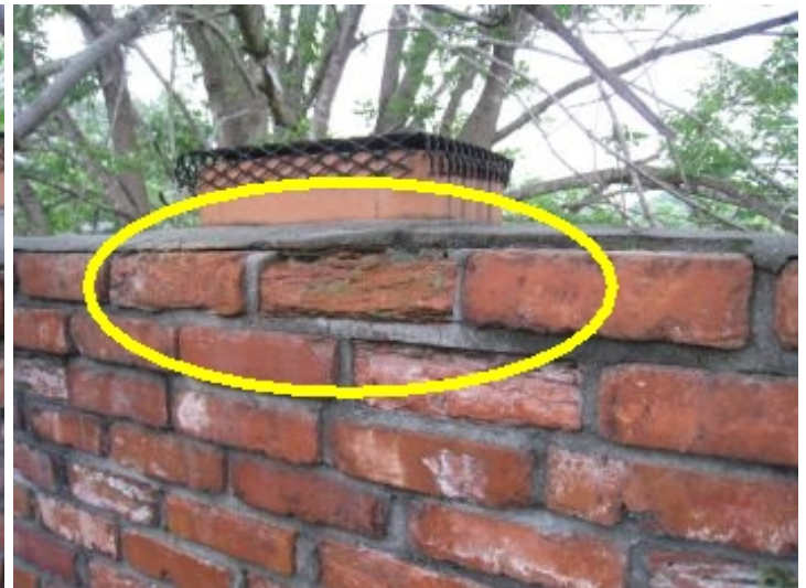
Deterioration at top of chimney
