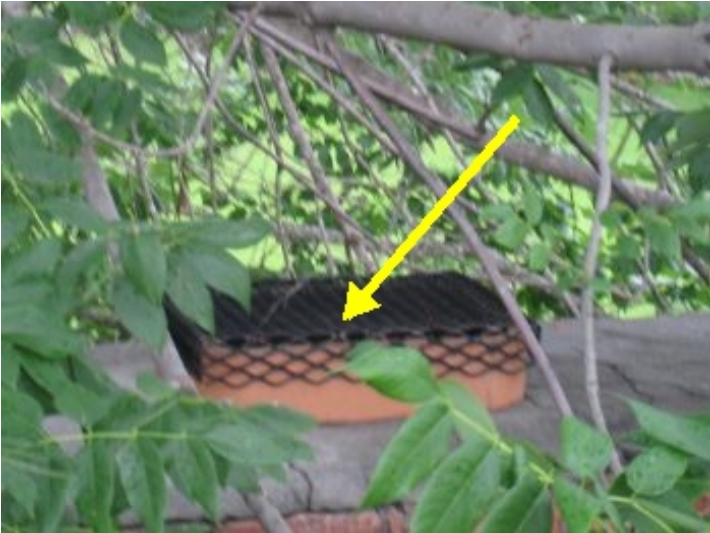
Missing chimney cap
