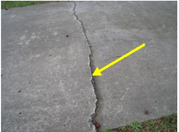
Crack in driveway
