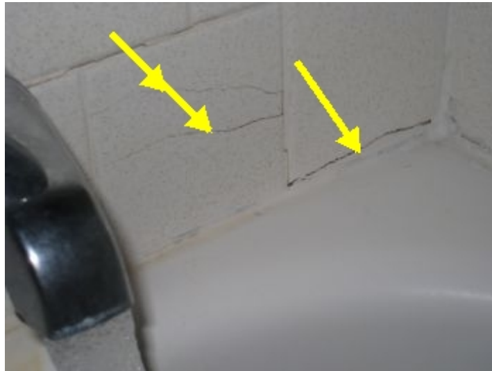
Broken tile at master bath tub
