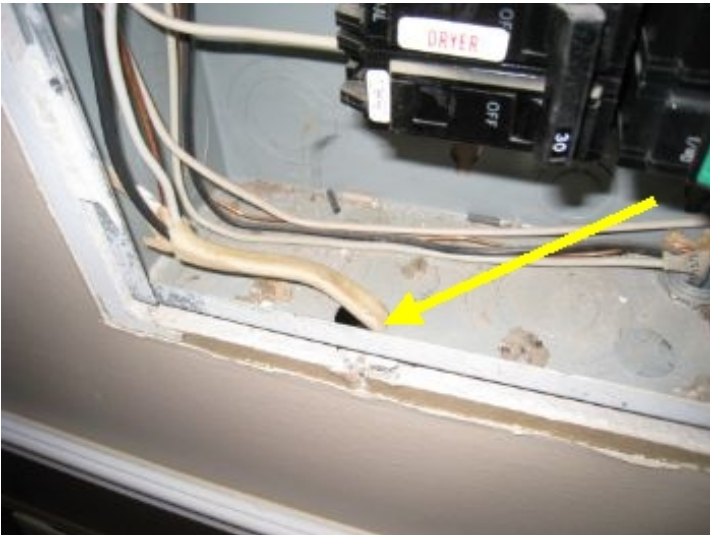
Missing bushing at cable entrance
