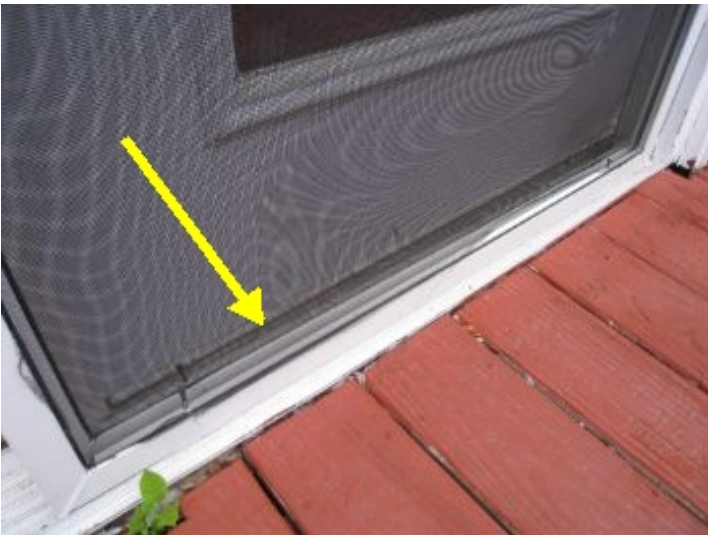
Damaged screens at back door
