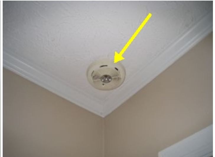
Smoke detector in dining room
