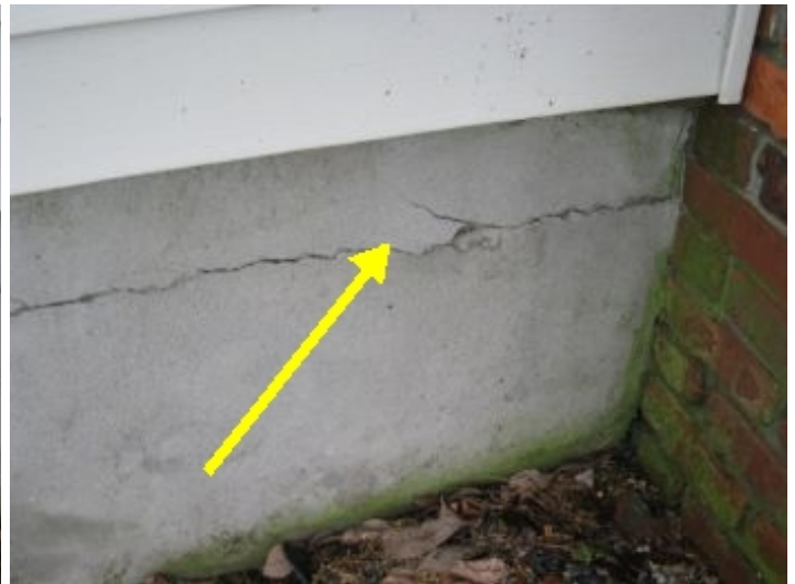
Minor foundation crack
