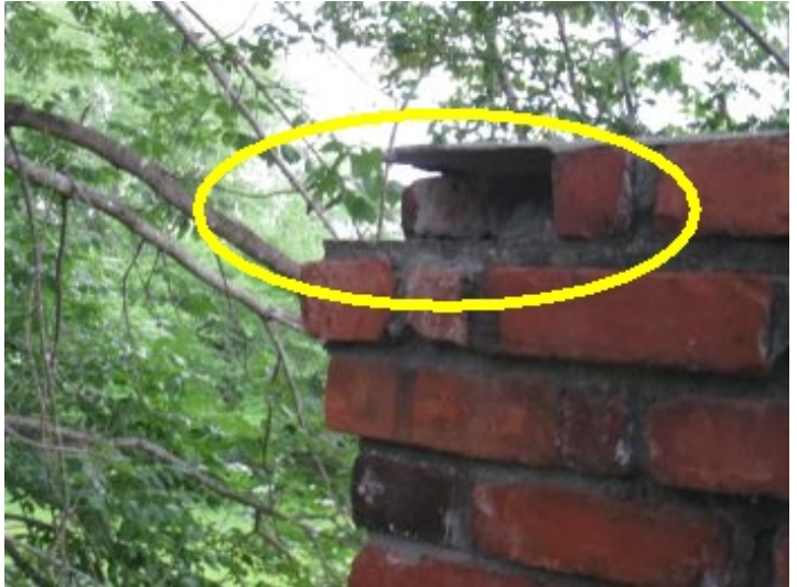
Missing bricks at top of chimney
