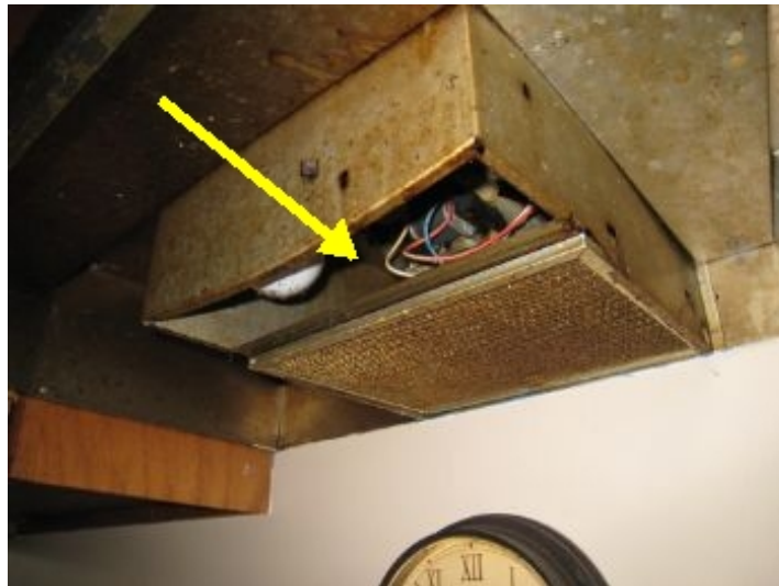
Missing cover for vent light
