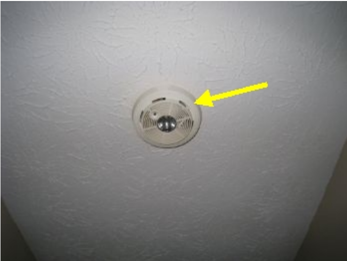
Smoke detector in hall
