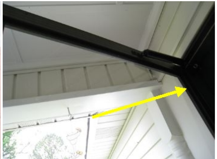
Loose glass panel in front storm door
