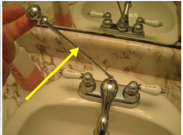
Loose pop-up stopper operator in hall bath
