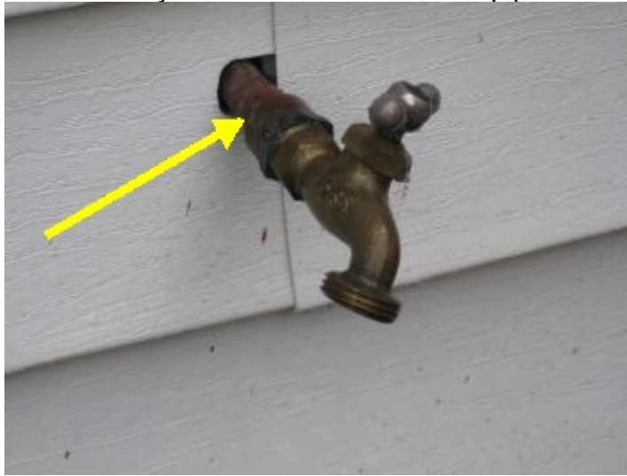
Unsupported hose bib
