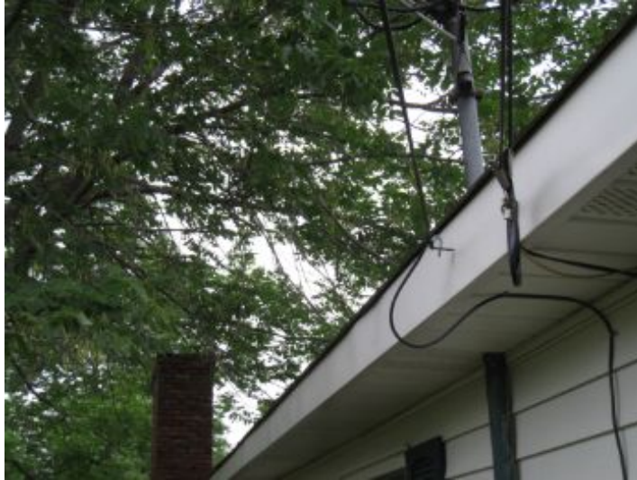
Tree overhanging roof
