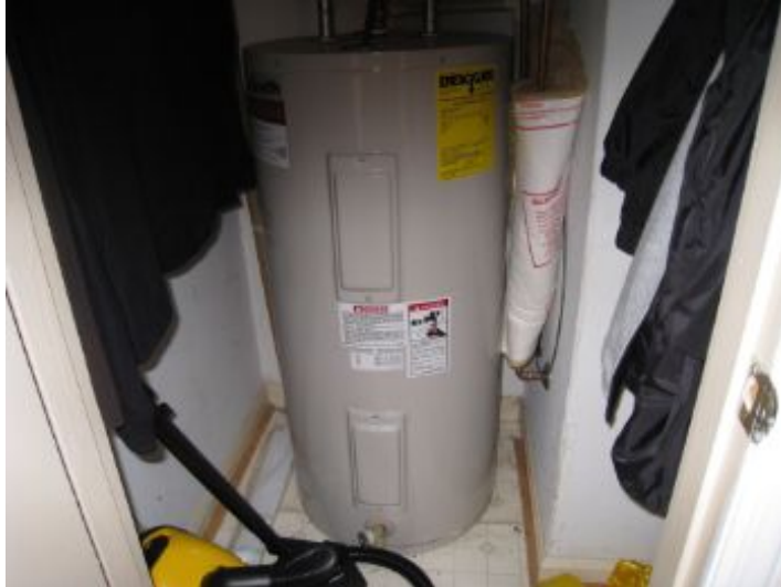
Water Heater in closet near front door
