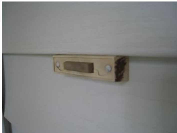
Broken doorbell button at front door
