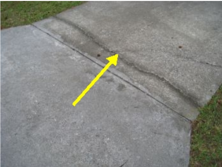
Crack in driveway
