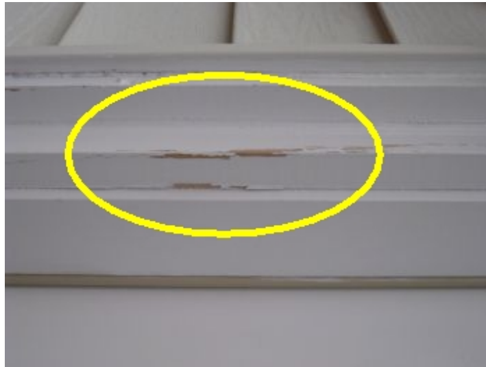
Failing paint around back door
