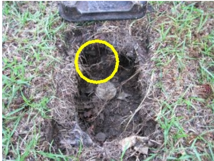
Water Meter and main water shut-off
